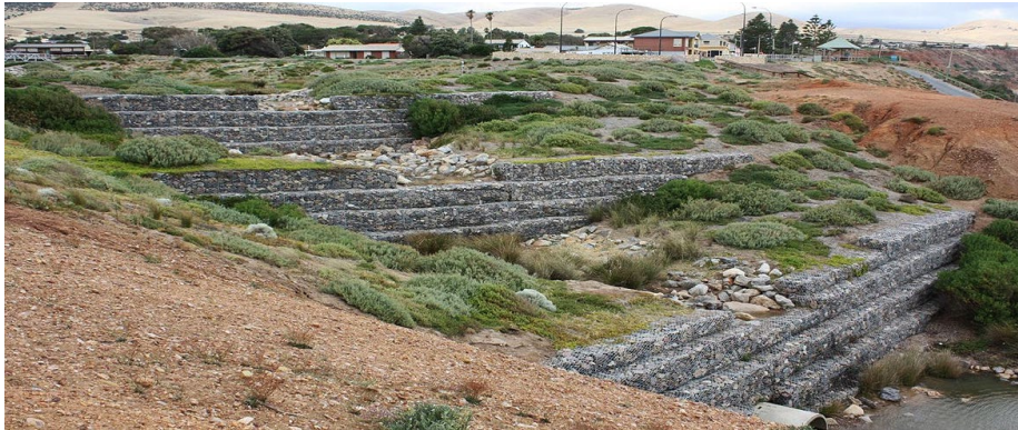
Above: Example of multi-stepped, multi-tiered grade control structure constructed using gabions, which are wireframe containers that have been filled with rocks
